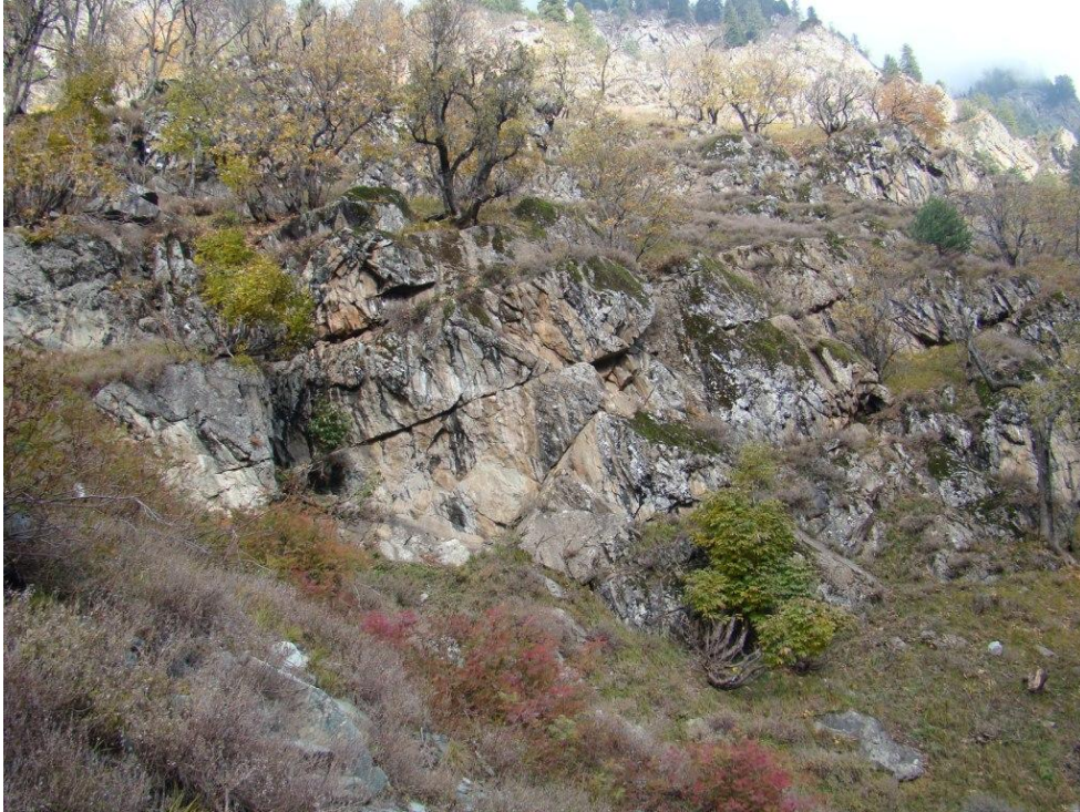
Fig. 27 A View of Joint along tunnel alignment, Joints run for more than 30 m.
